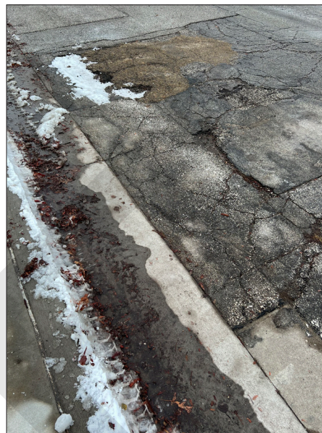
Figure 4.5 – Example of poor pavement conditions due to freeze/thaw cycle, Rock Island, Illinois
